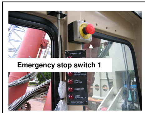
Installed in the operator's room
